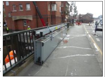
One of the new stop planks
